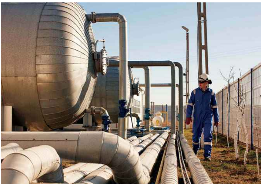
Above Water and gas separation facility, Ticleni oil field, Romania.
